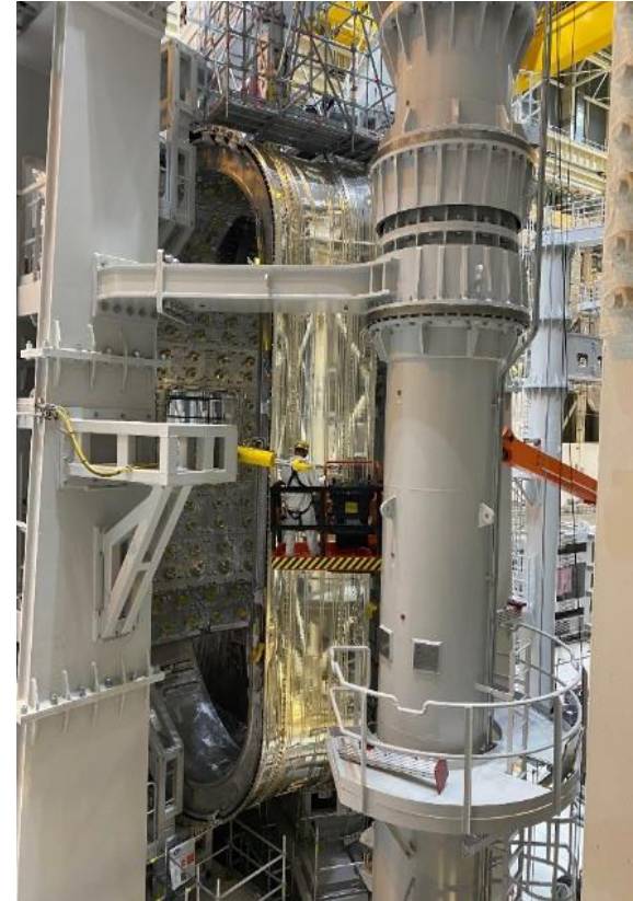
VVTs #6: Insulation Test
