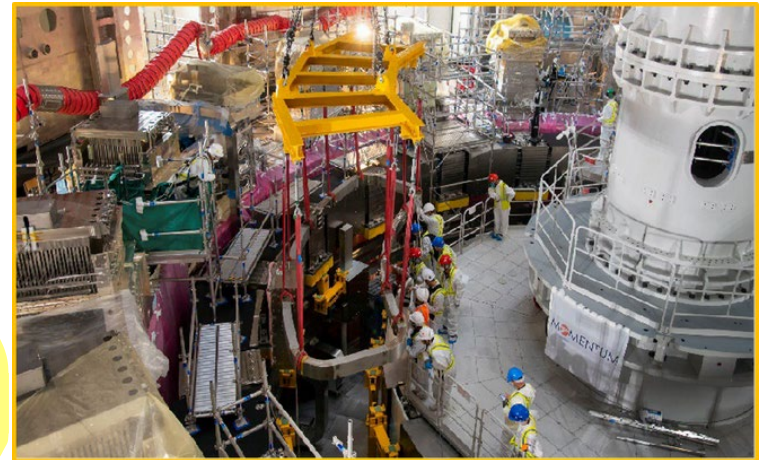
Bottom correction coils installed
